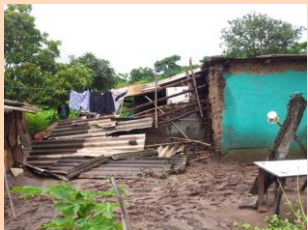
Rainstorm effected 200 homes in Redcliff (Query)Community
